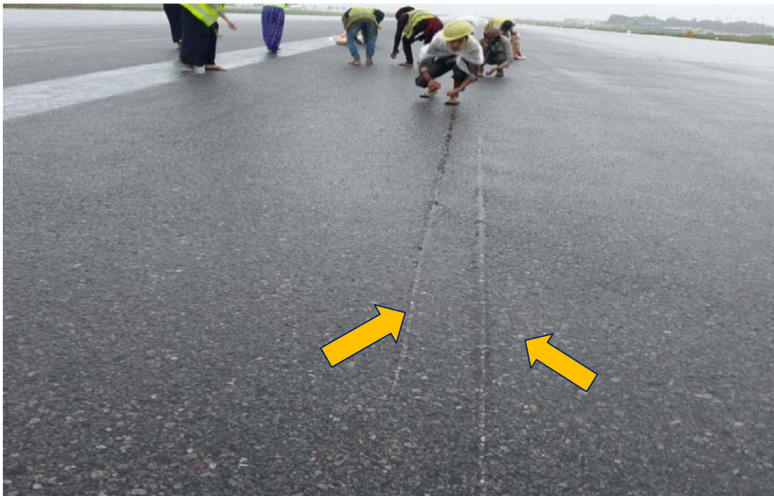
Figure (7) Impact marks on the runway
