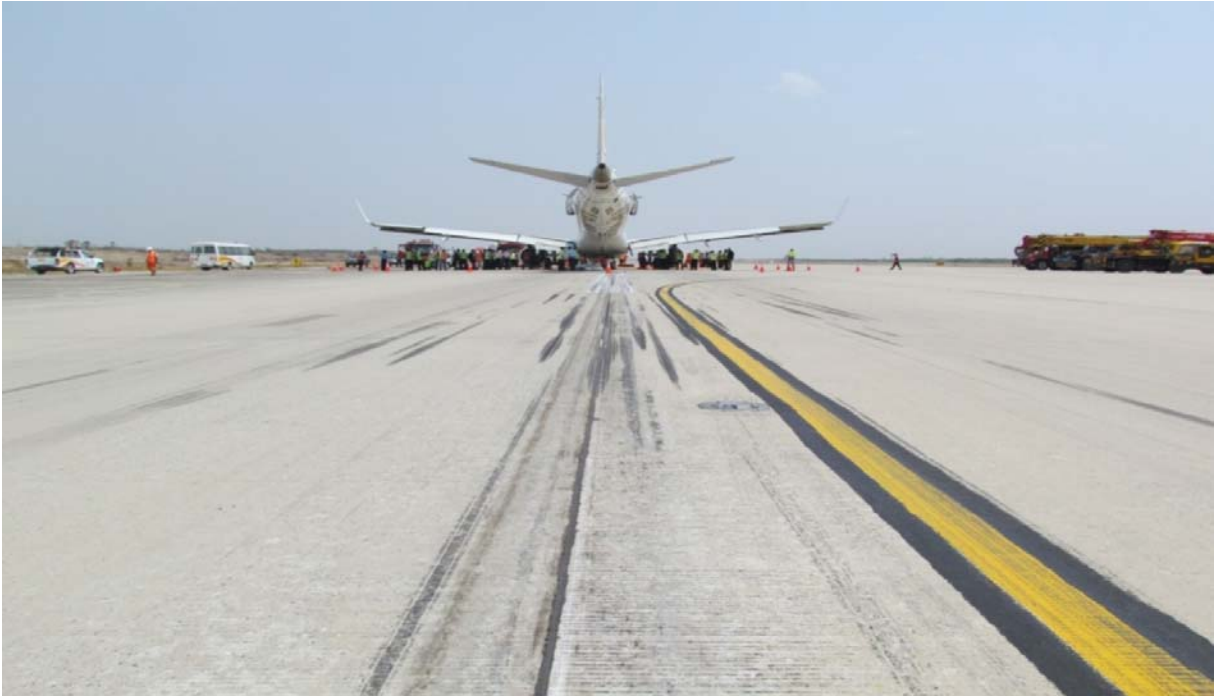
Figure (8) The Impact Marks on the runway
