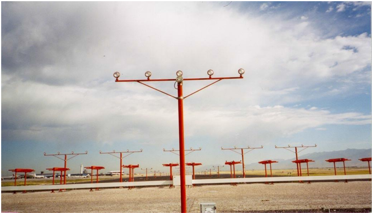
Figure 4-3. Approach lighting towers — fibreglass tubular poles
