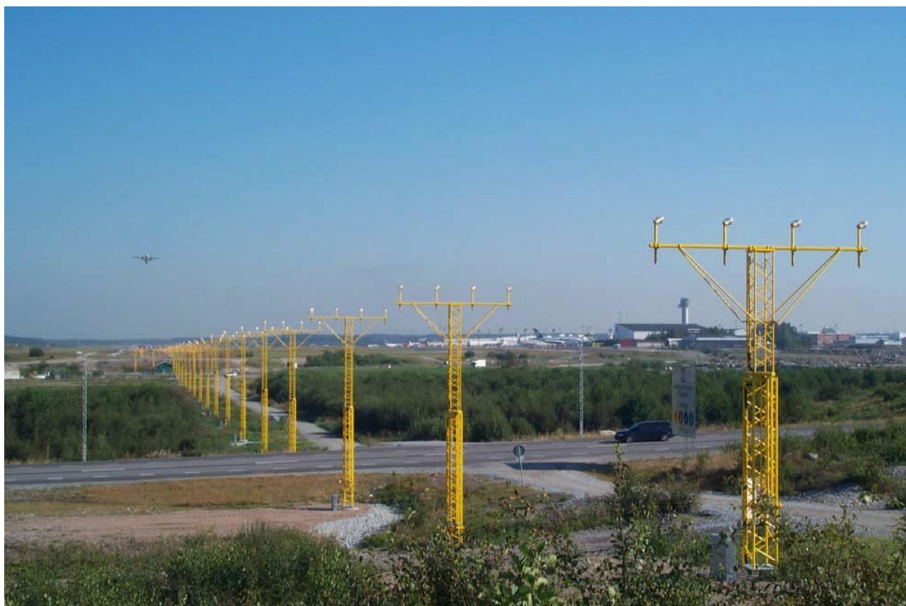
Figure 4-2. Approach lighting towers — fibreglass lattice structures
