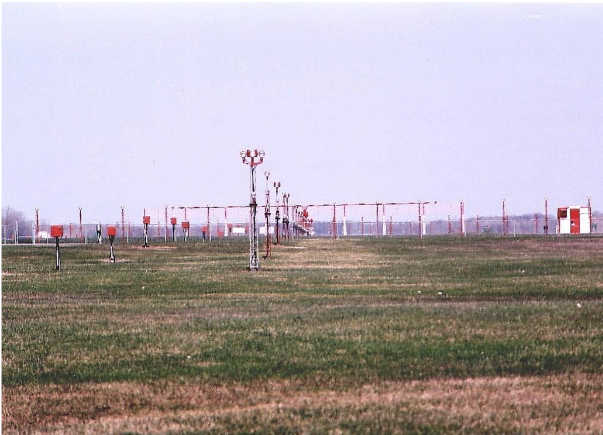
Figure 4-4. Approach lighting towers — aluminium lattice structures
