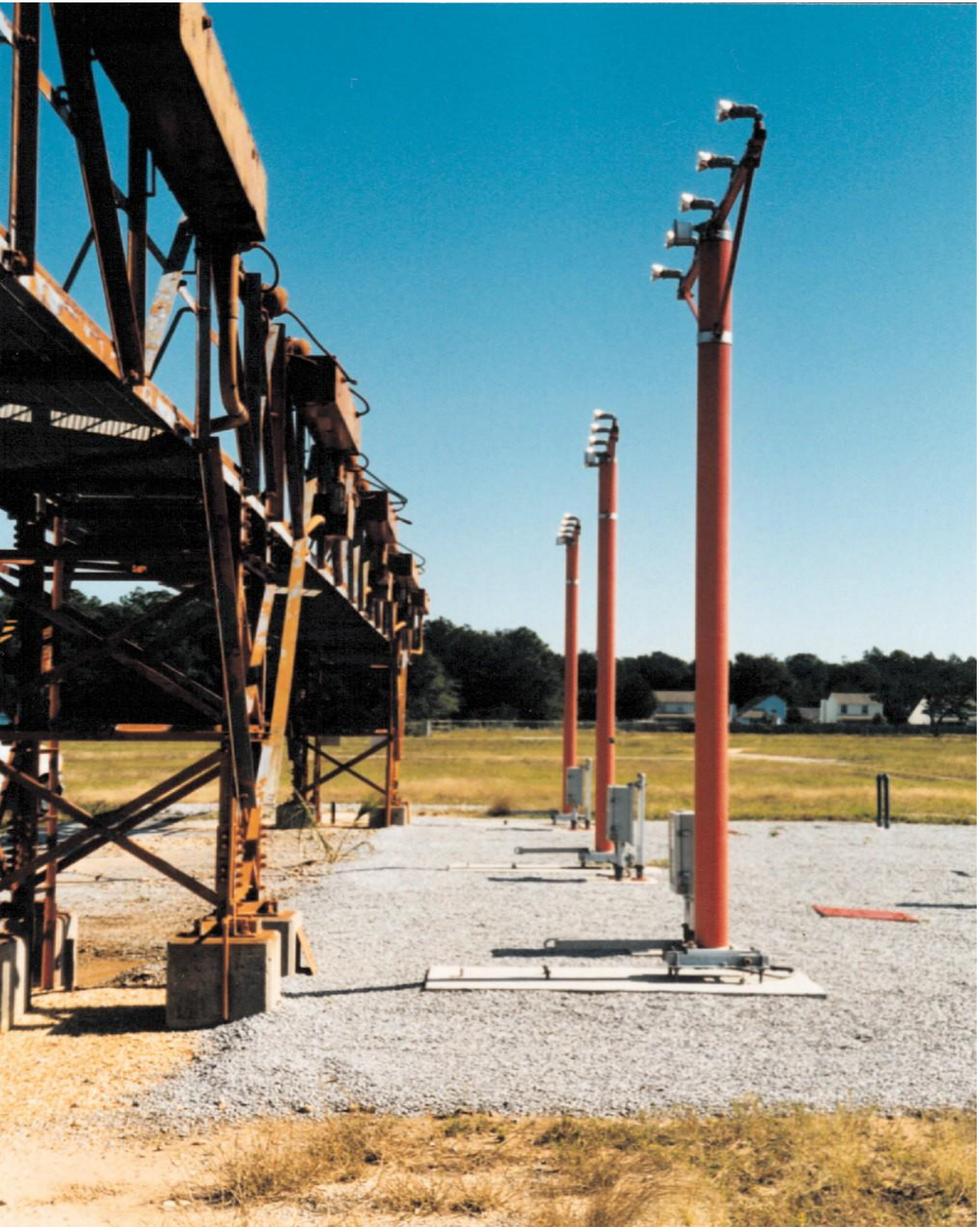
Figure 4-6. Approach lighting station of rigid design (Left) being replaced by new frangibility structure (right)
