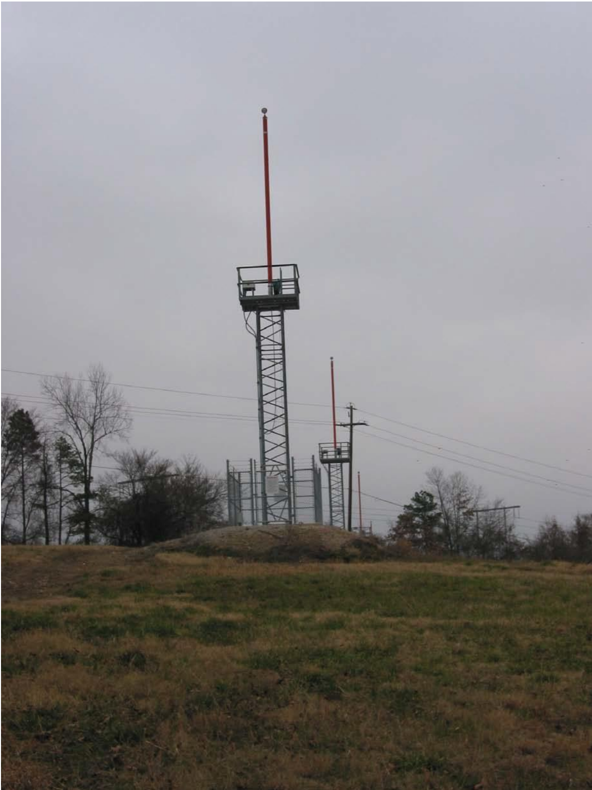
Figure 4-7. Fiberglass tubular pole on rigid structure
