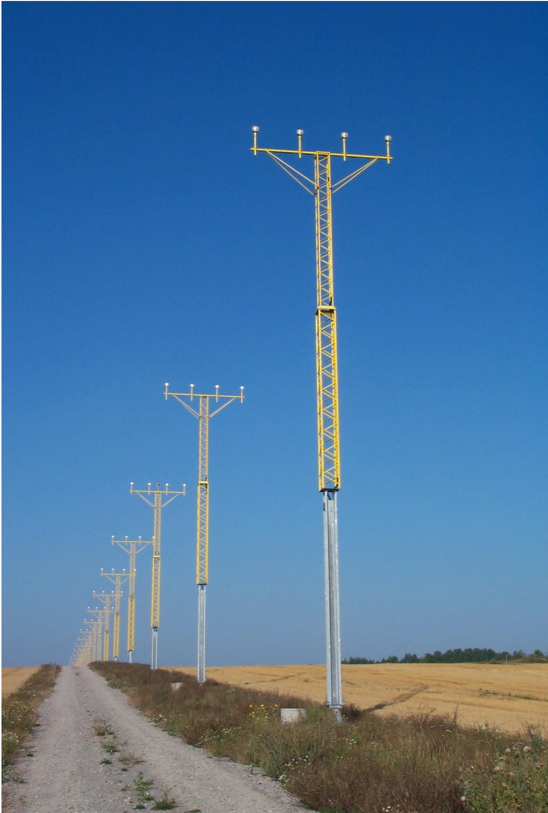
Figure 4-8. Fiberglass Approach lighting towers on rigid supporting structure
