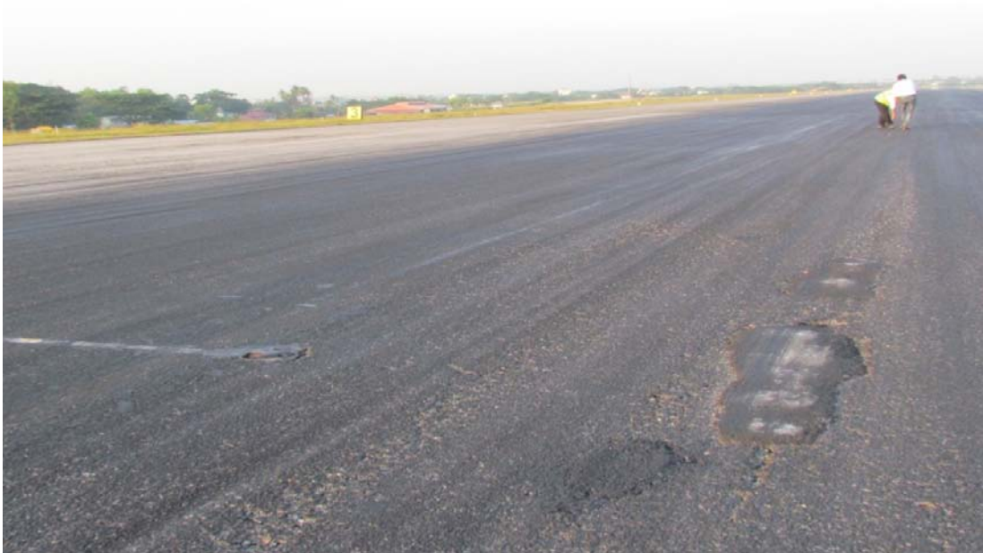
Figure (5) Scrape marks on the runway
